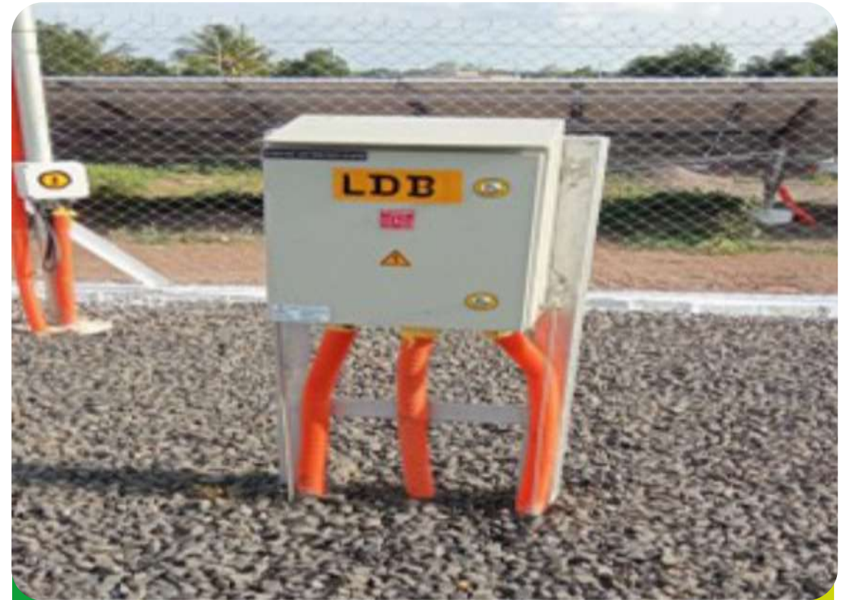
Light Distribution Box
