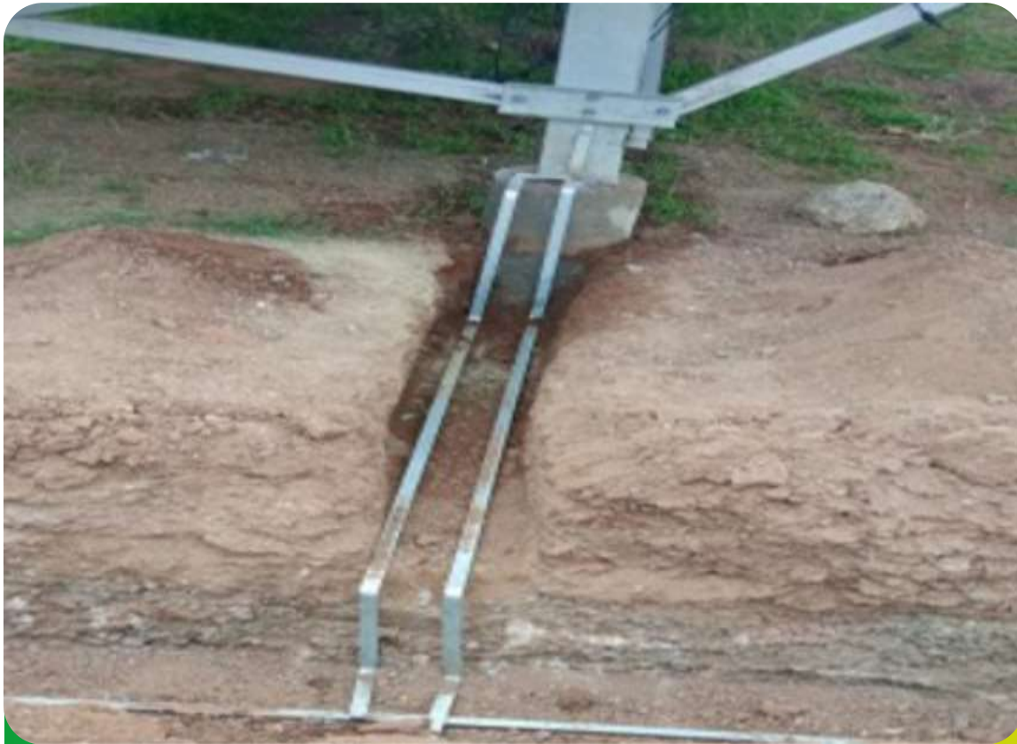
Dc Earthing With Perfect Bend & Cross Joint
