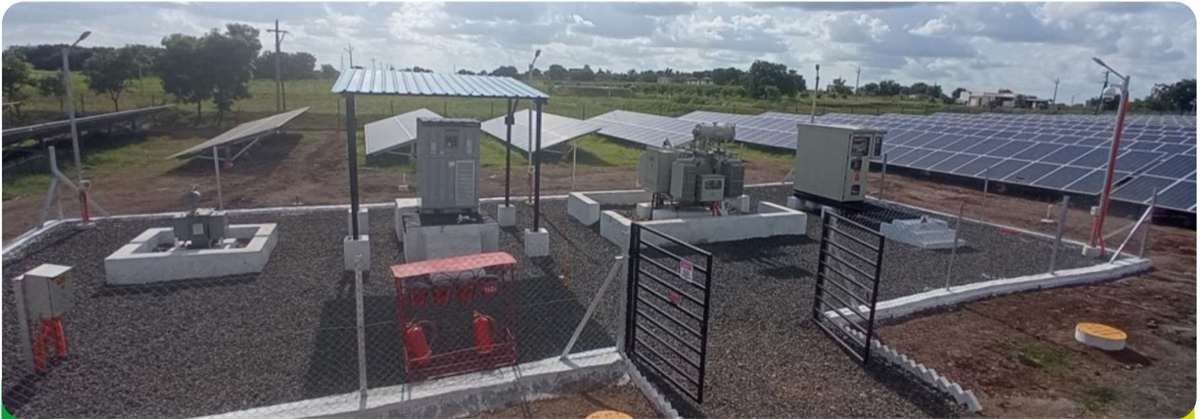
Clean Switchyard After Housekeeping
