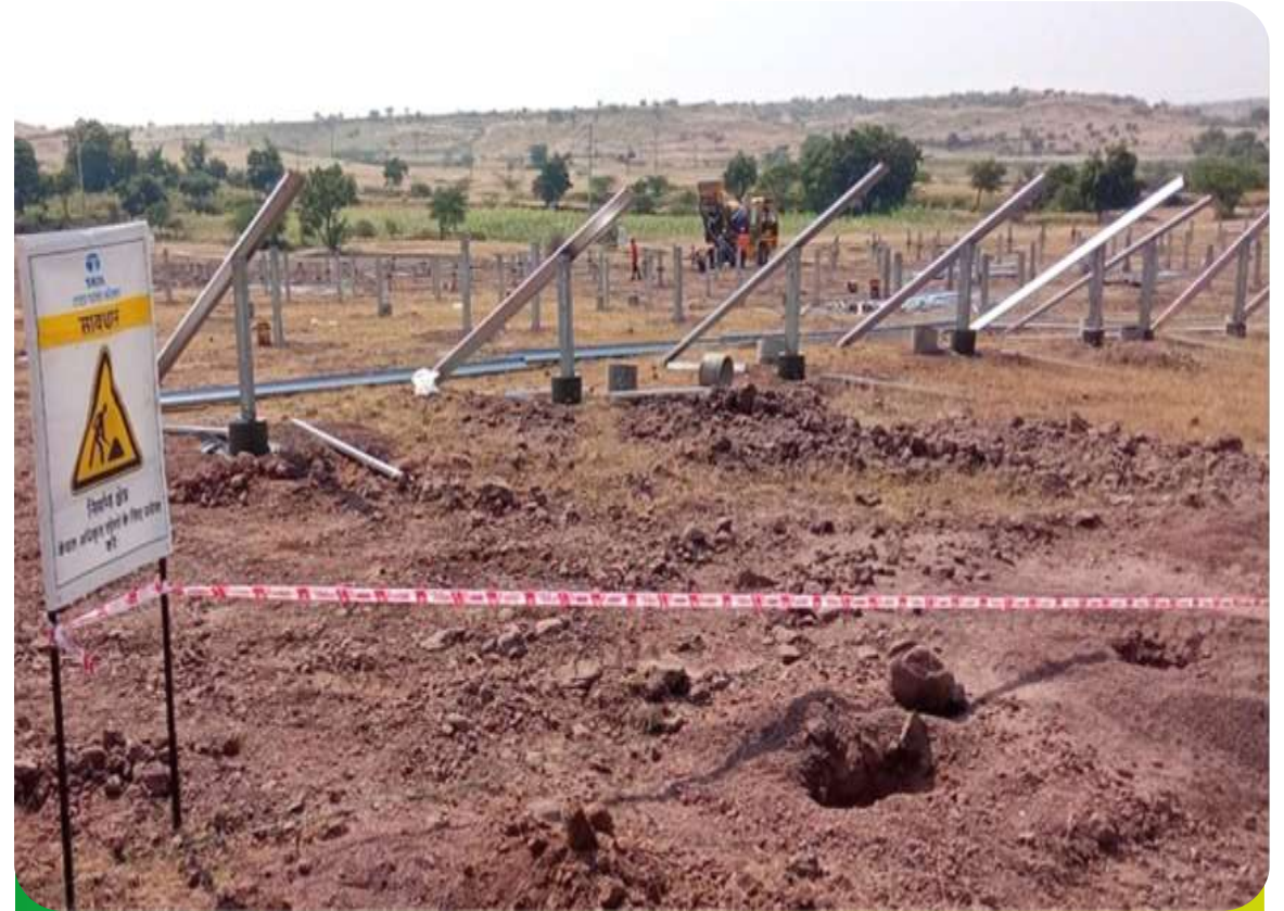
Mms Work With Safety, Caution Warning
