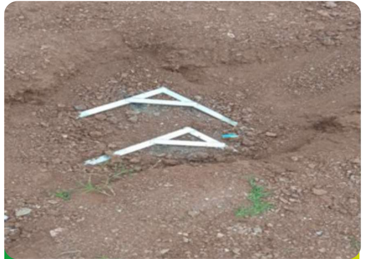
Dc Earthing With Perfect Bend & Cross Joint
